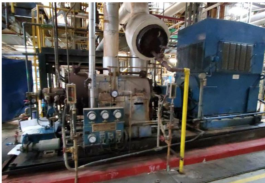
Figure 1: Unit 1 Boiler Feed Pump East
